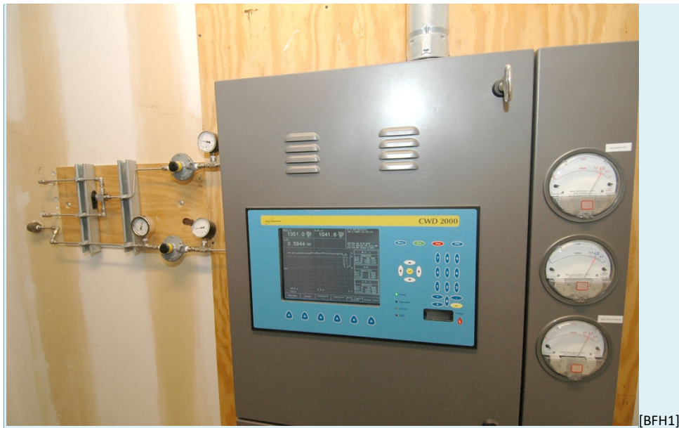
Figure 1: Combustion Calorimeter Mounted to Wall in 1 Megawatt Shed
