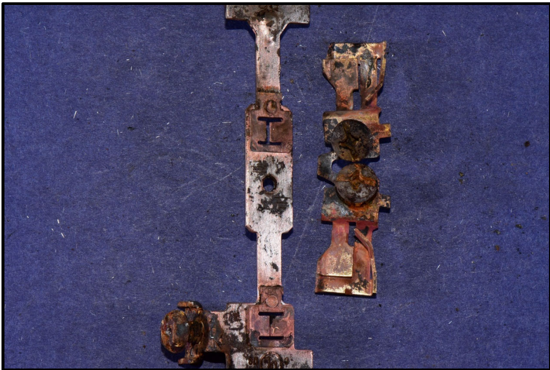
Figure 94. Power rail and ground yoke from Receptacle 13-B
