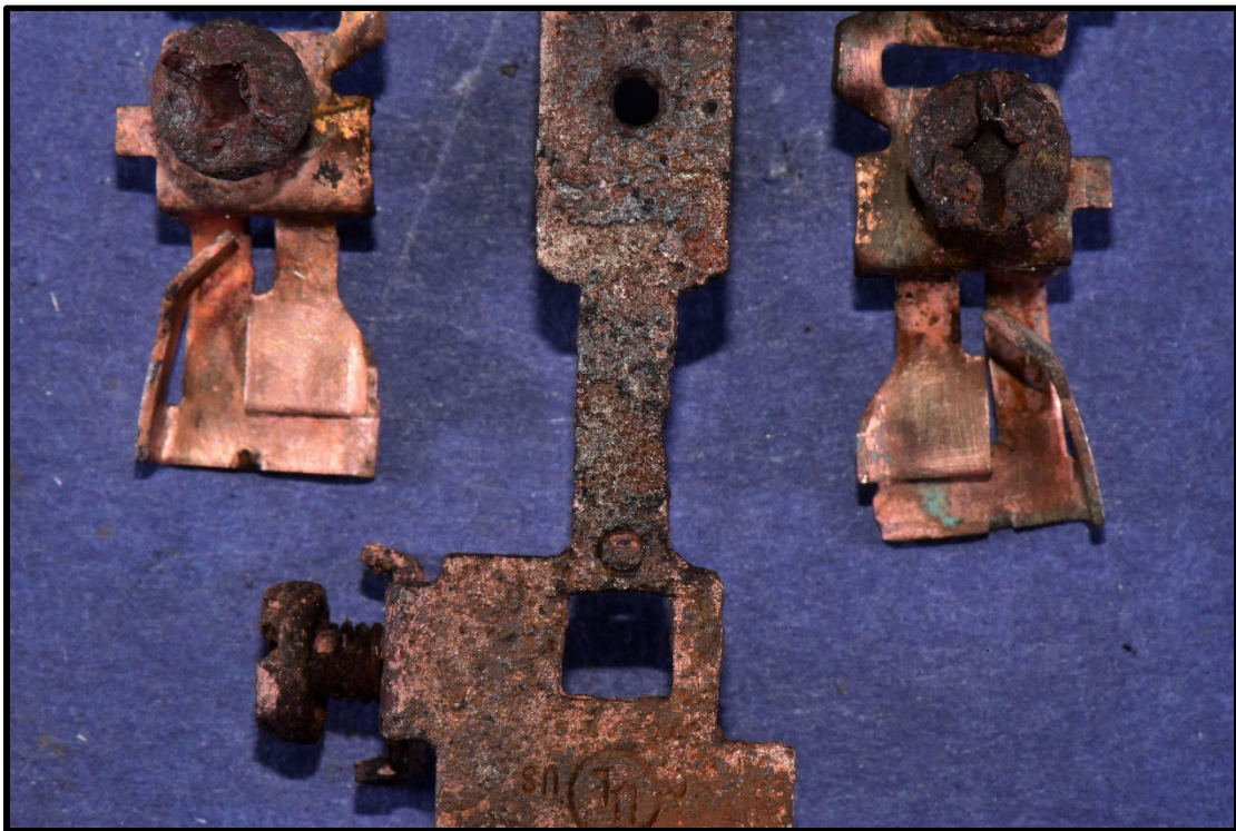
Figure 45. Power rails and ground yoke from Receptacle 13-S
