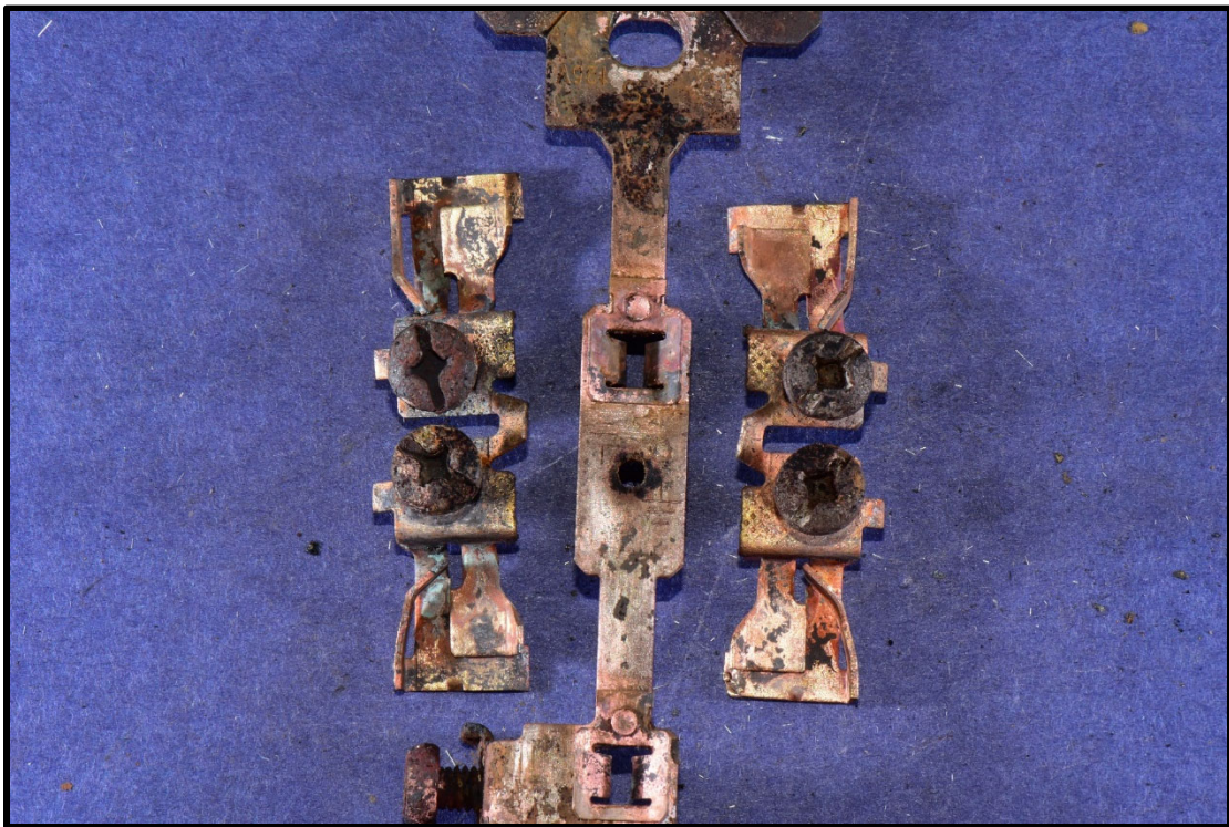
Figure 98. Power rails and ground yoke from Receptacle 16-A
