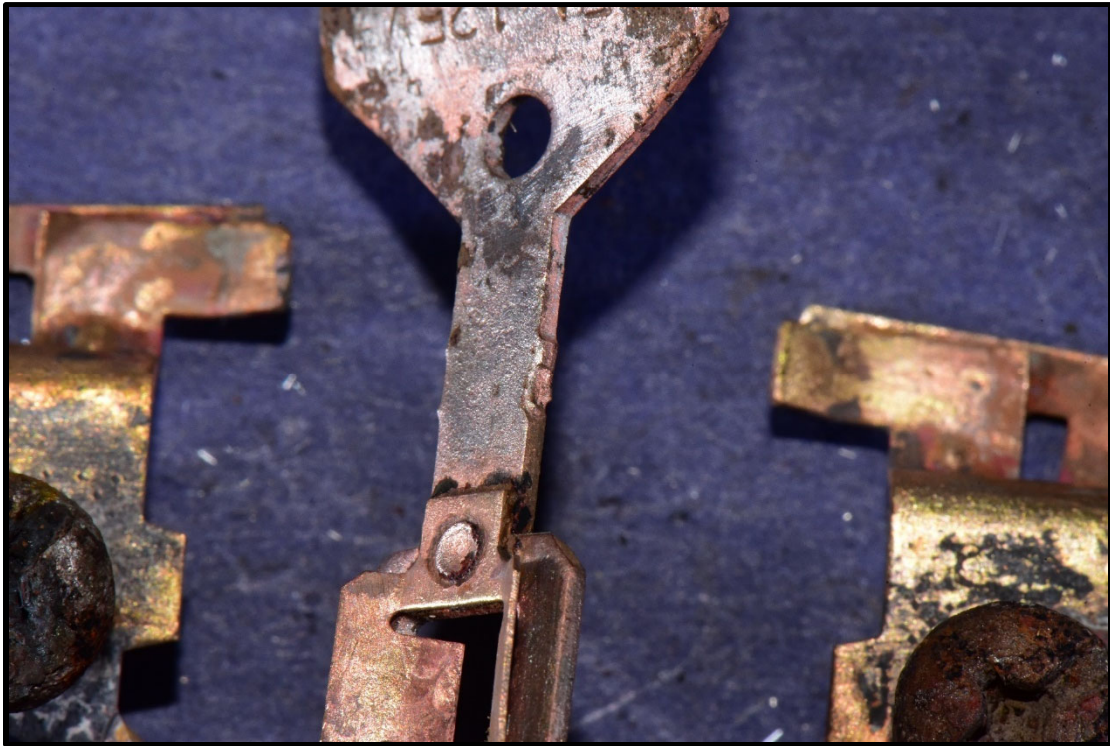
Figure 103. Power rails and ground yoke from Receptacle 17-B
