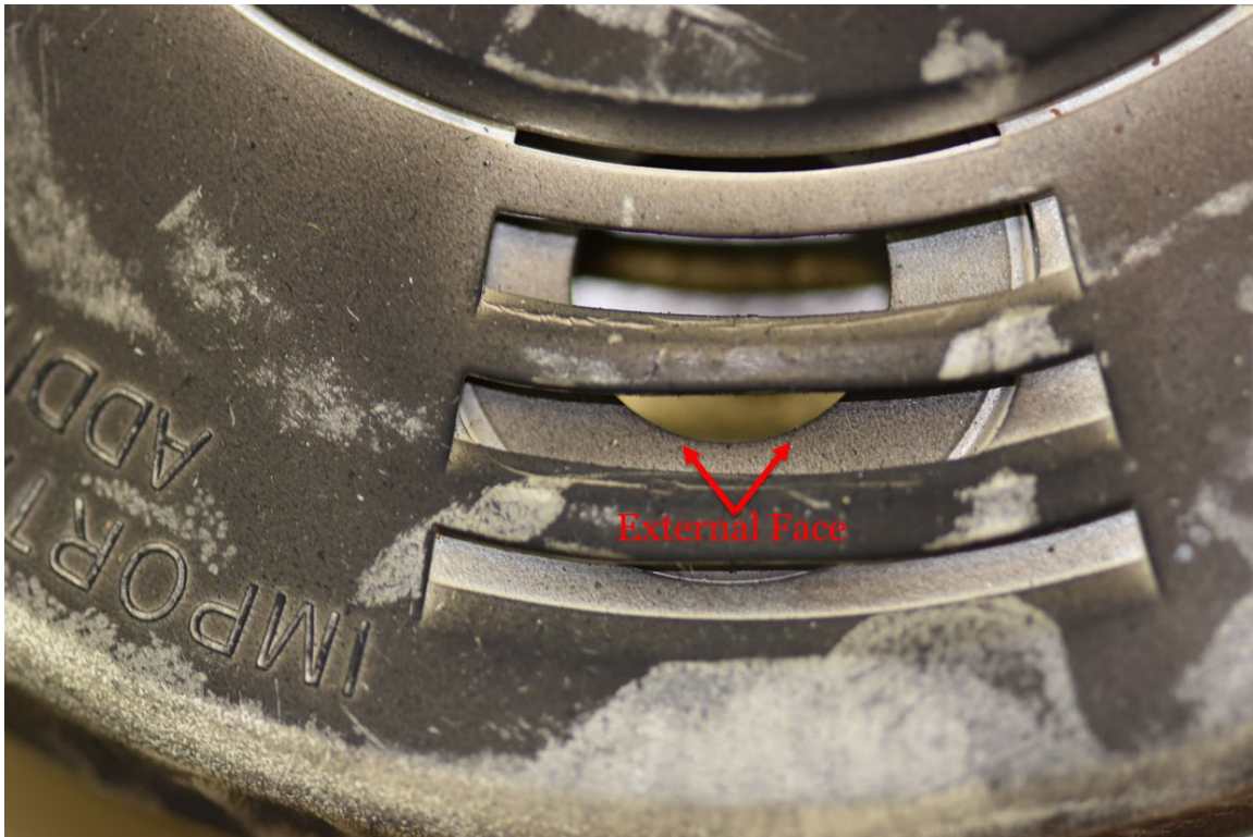
Figure 40. Example of an exposed smoke alarm without ESD on the external face of the horn chamber. Note the relatively uniform distribution of soot on all exposed surfaces.
