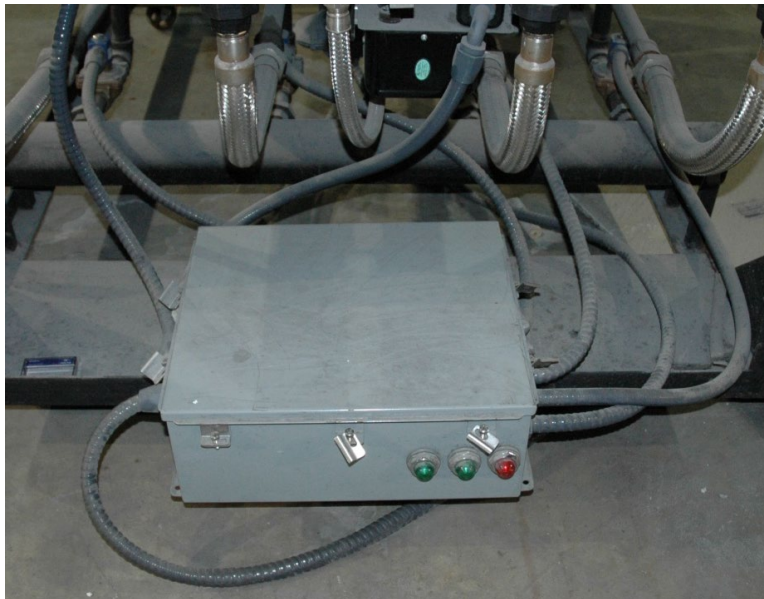
Figure 12 - Gas burner electrical circuit box with LED indicator lights
