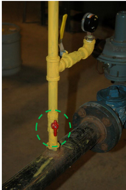
Figure 2. Combustion Calorimeter Connection to the Natural Gas Supply Line; Red Valve Shown in the “ON” Position.
