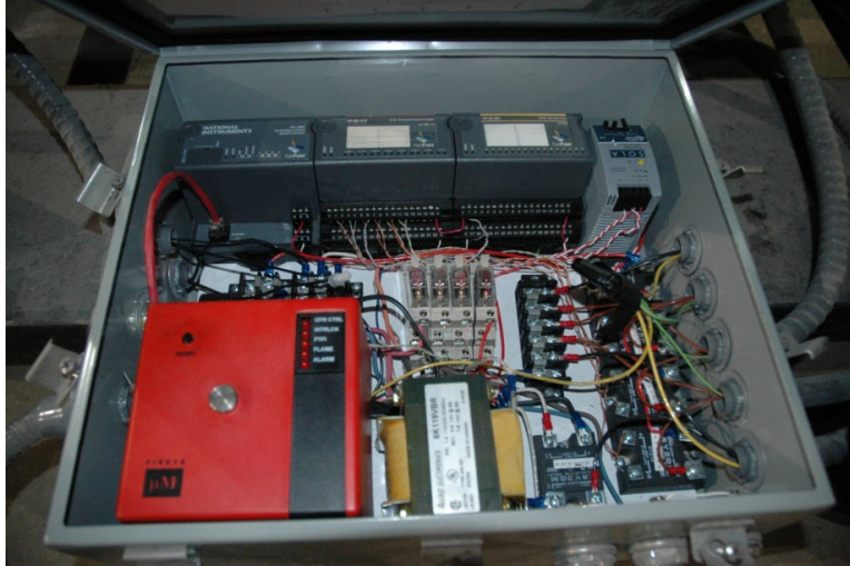
Figure 11 – Gas burner electrical circuit box containing Fireye (bottom left corner), FieldPoint Module (top) and solid state relays (right)
