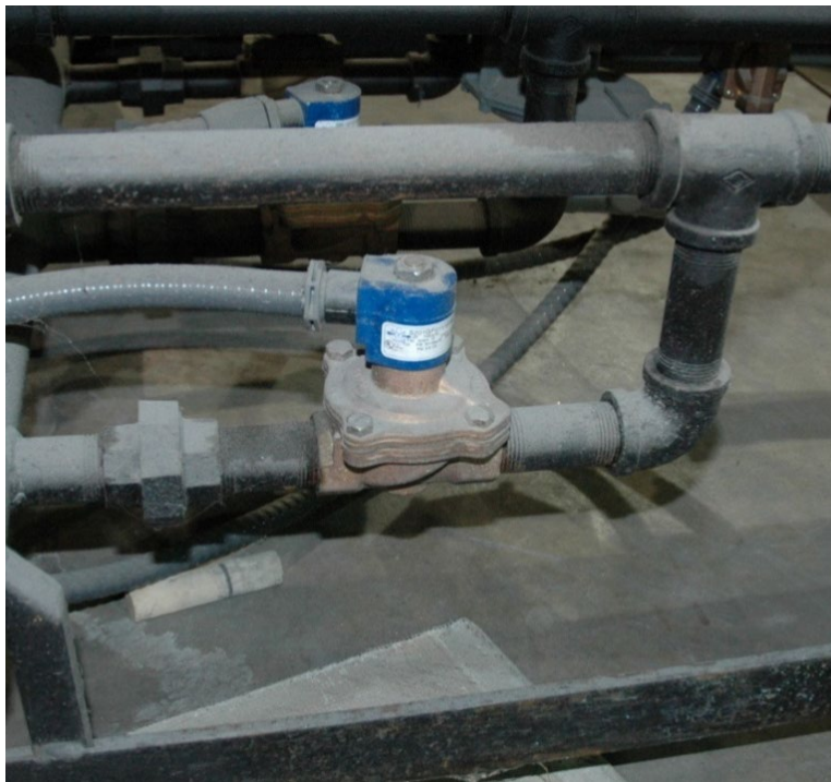
Figure 9 – Solenoid valve connected to tube bank "4"
