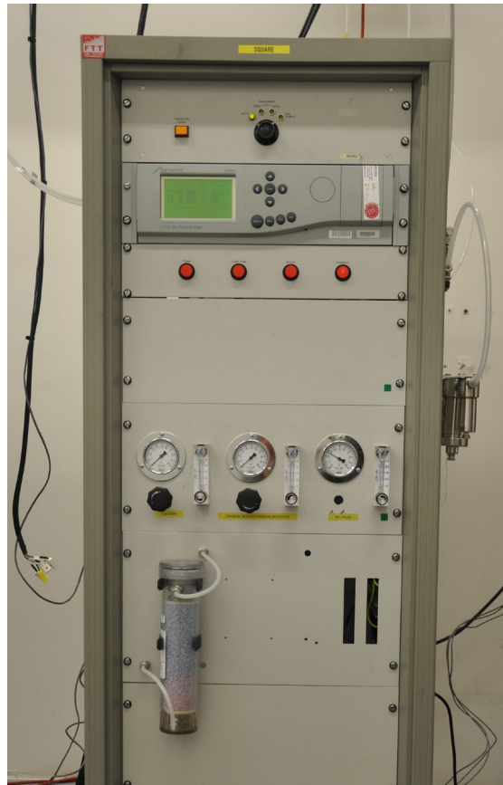
Figure 6: Photo of the 4 MW FPC gas analysis rack
