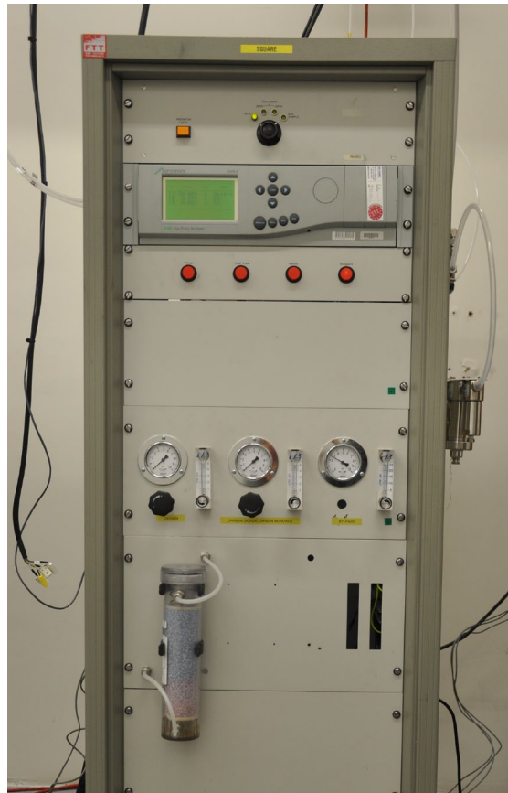
Figure 6: Photo of the 1 MW Square FPC gas analysis rack
