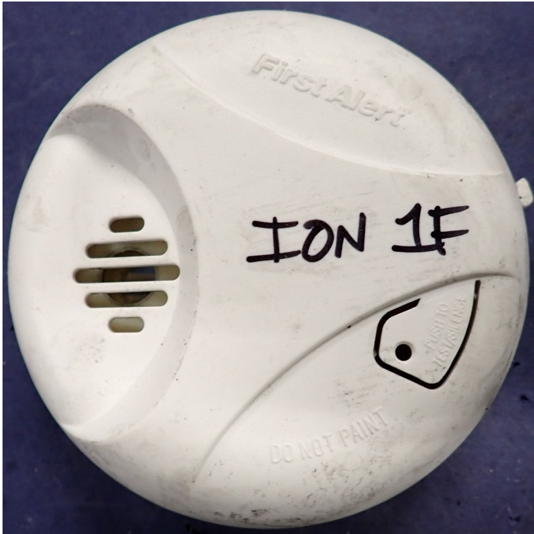
Figure 7. Example of a smoke alarm with sufficient, overall depositions of products of combustion. Note the general, relatively uniform, soot staining on the entire surface of the alarm cover.
