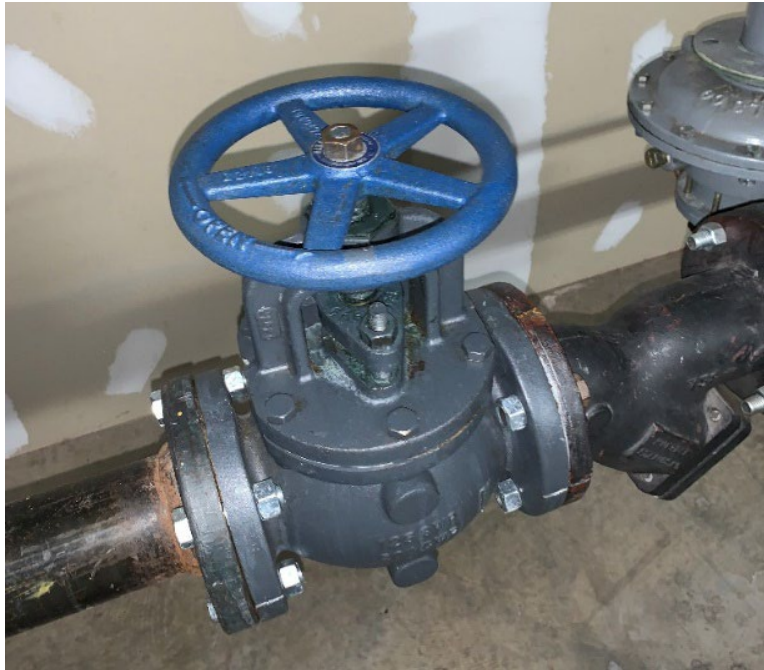
Figure 2 –Manual Shutoff Valve for Mezzanine Gas Train
