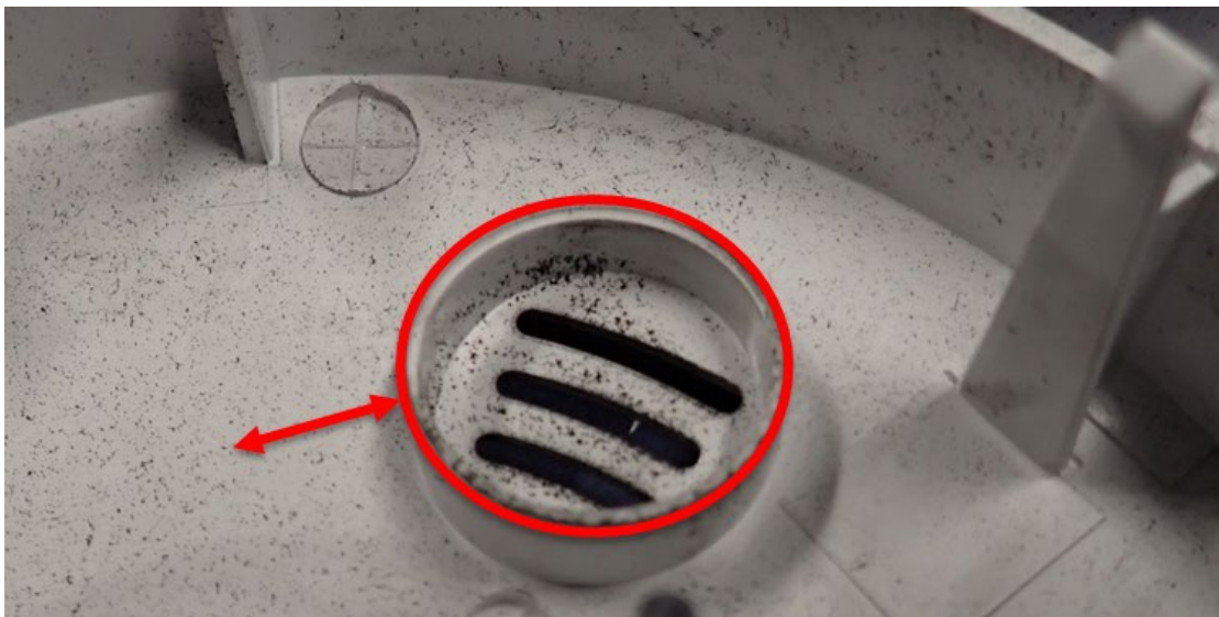
Figure 24. ESD observed within the alarm cover inset for the horn chamber. Note the differential soot deposition (more) with relative to that observed on adjacent surfaces.
