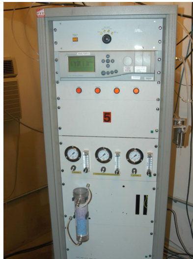
Figure 2. Rack housing of Servomex Analyzer
