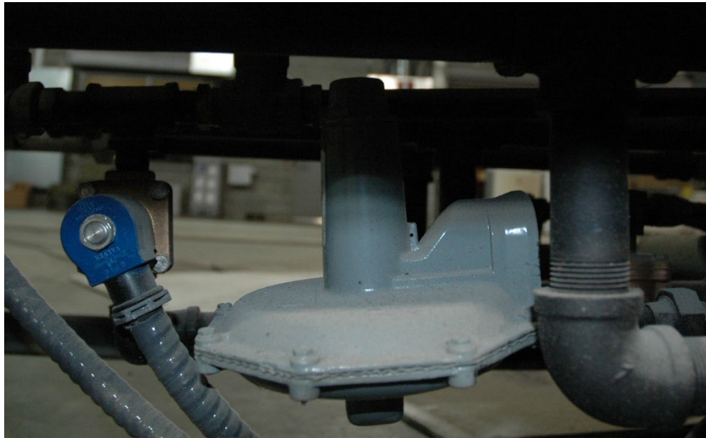
Figure 10 – Pressure regulator (center) and solenoid valve (left) for gas burner pilot tube
