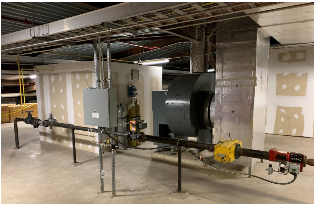
Figure 1 - Gas Train in Mezzanine
