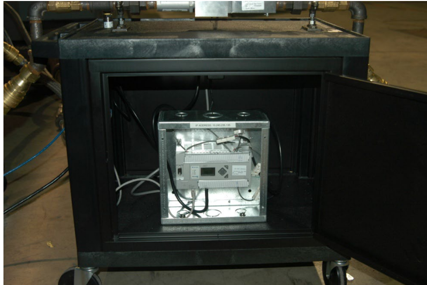
Figure 5. Allen Bradley MicroLogix 1400 PLC inside Gas Cart
