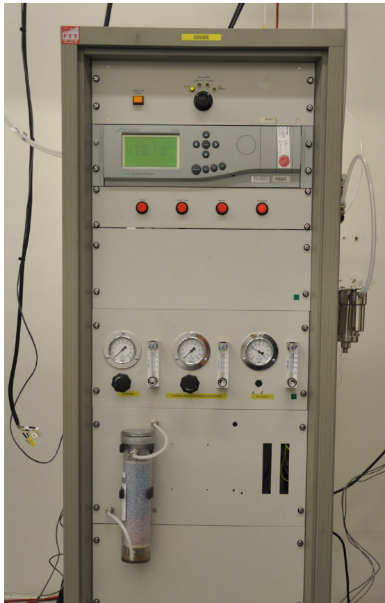
Figure 6: Photo of the 1 MW Round FPC gas analysis rack
